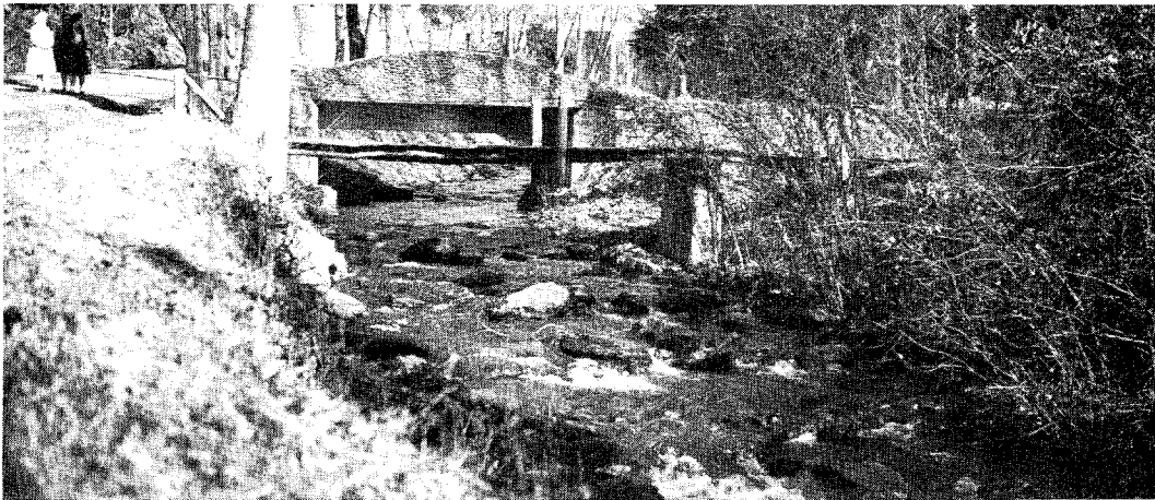
Footbridge and Lookout Road bridge, Miles 2.43 and 2.44, downstream side. Part of the Montreat Dam appears in top center of picture.
