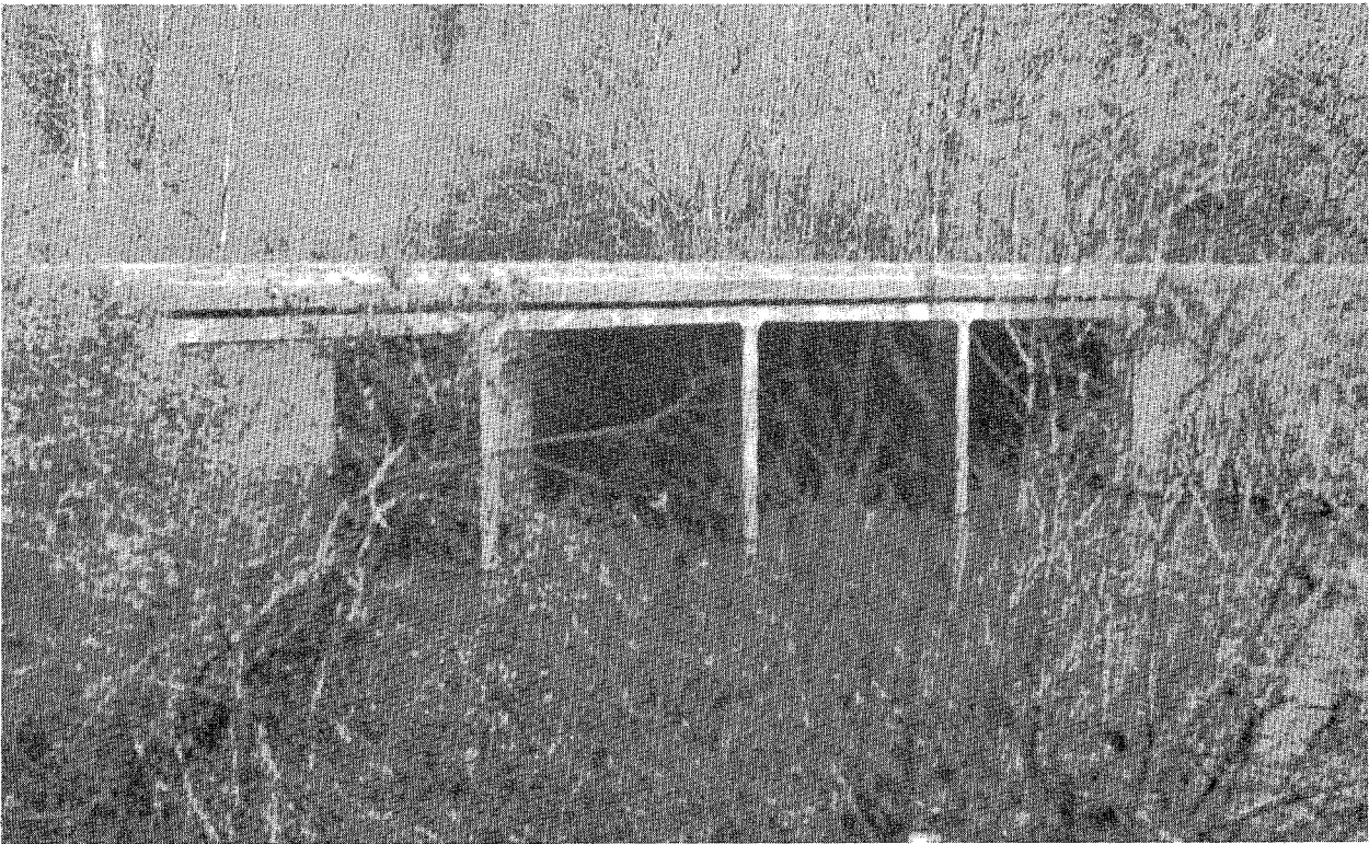
Figure 6. --BRIDGES ON WEST FORK FRENCH BROAD RIVER
